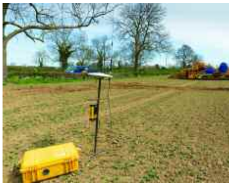
Installation equipment hasn't changed much since the 1980s, apart from more sophisticated levelling equipment and greater use of GPS.
