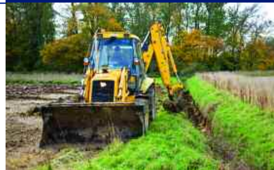
The ditch may have become silted and blocked the pipe, but consider the environmental implications of managing ditches.
