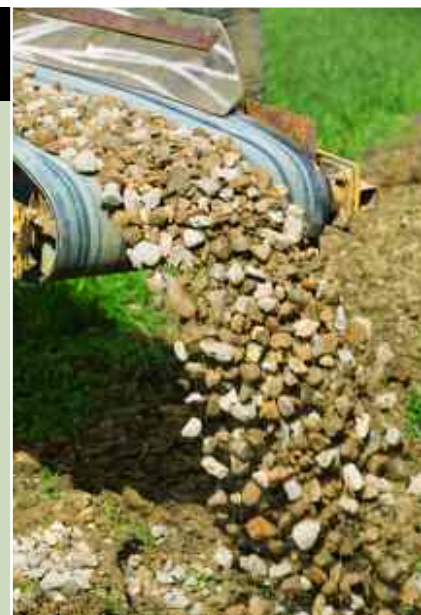
The backfill is a costly addition but the performance of drains on clay soils soon slows up if it's left out.
